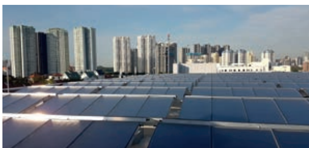
Extensive solar cooling system in Singapore
